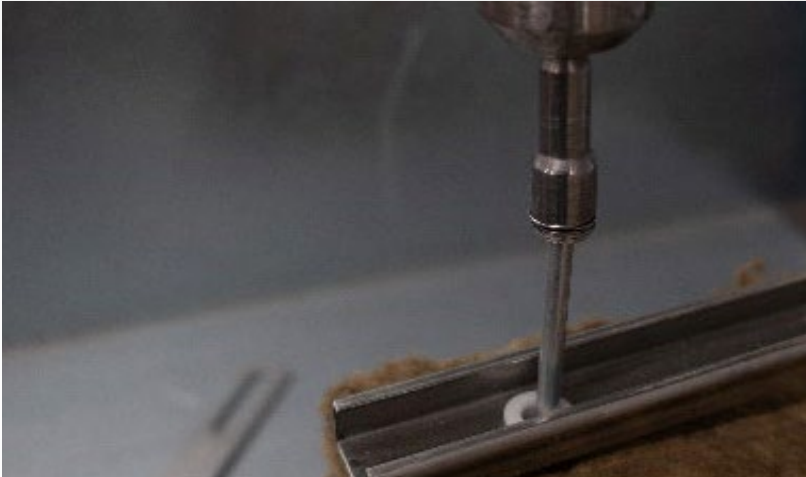
Figure 12 - Installation of fasteners for retention of wall-tie system to concrete or masonry
